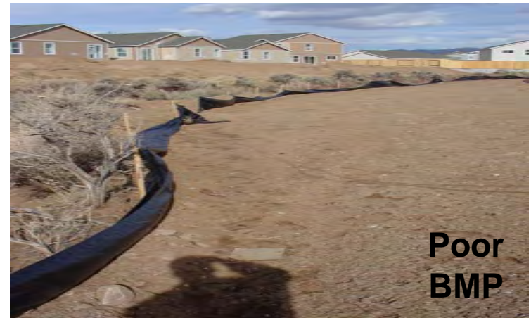
Poorly maintained fence
