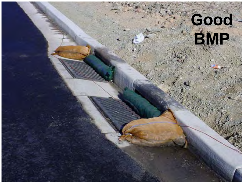
Effective drain inlet BMPs
