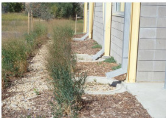
DOWNSPOUTS IN BOULDER
