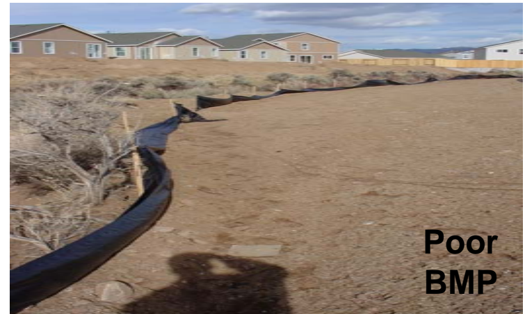
Poorly maintained fence
