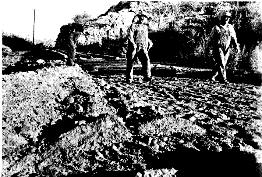
Figure 7 – Repair of railroad damage due to flooding in the Narrows between upstream limit of study and Glendale during the flood of 1960.
