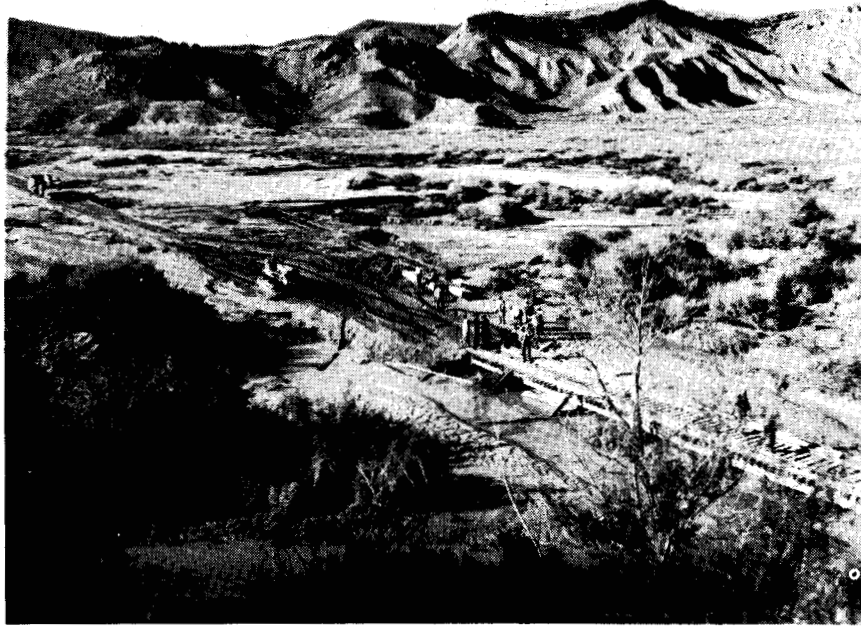
Figure 13 — Railroad embankment washout being repaired after the 1960 flood. The site is north of the study area and about 10 miles north of Overton.
