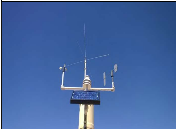
Photo 5: View of instrumentation atop of Rain Gauge, North Site.
