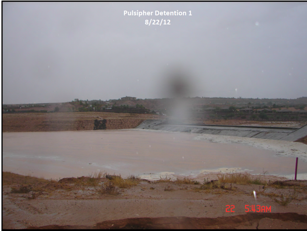
Pulsipher Wash DB captured 6.5 feet of runoff
