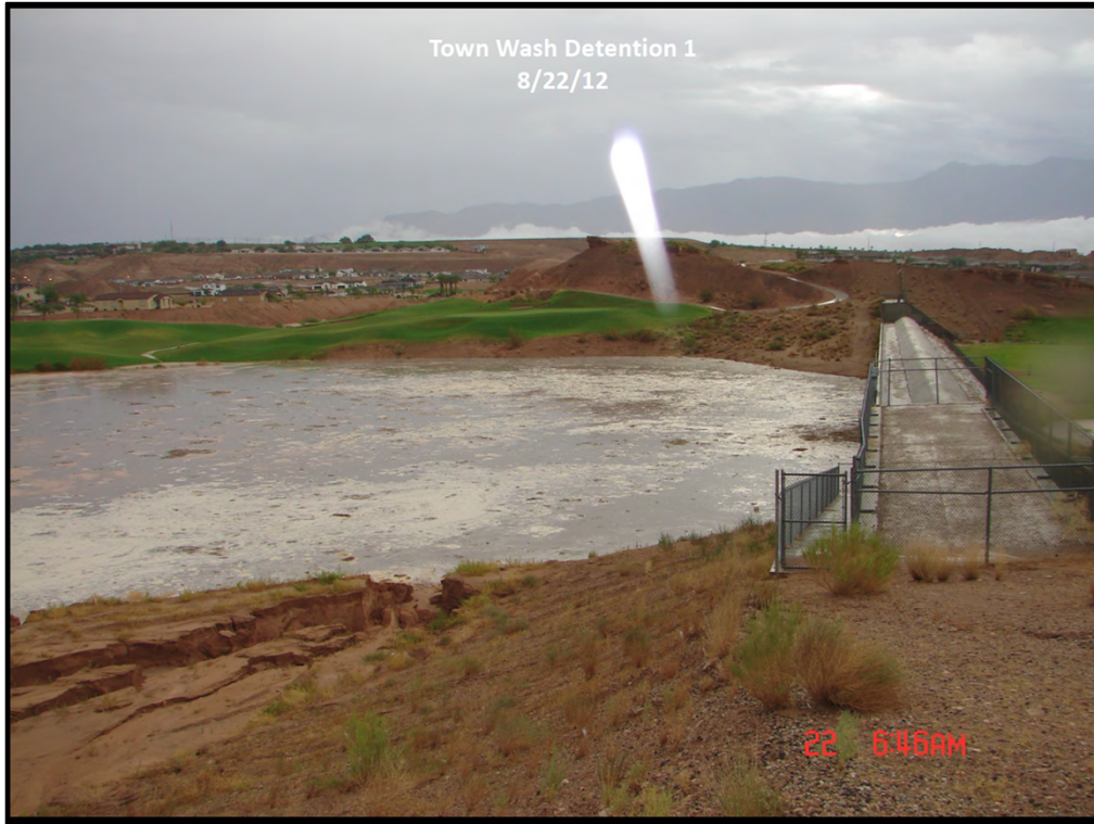
Here are a few photos of the aftermath of this storm. Jim Wilson (aka Town Wash) DB impounded 8.5 feet of runoff.
