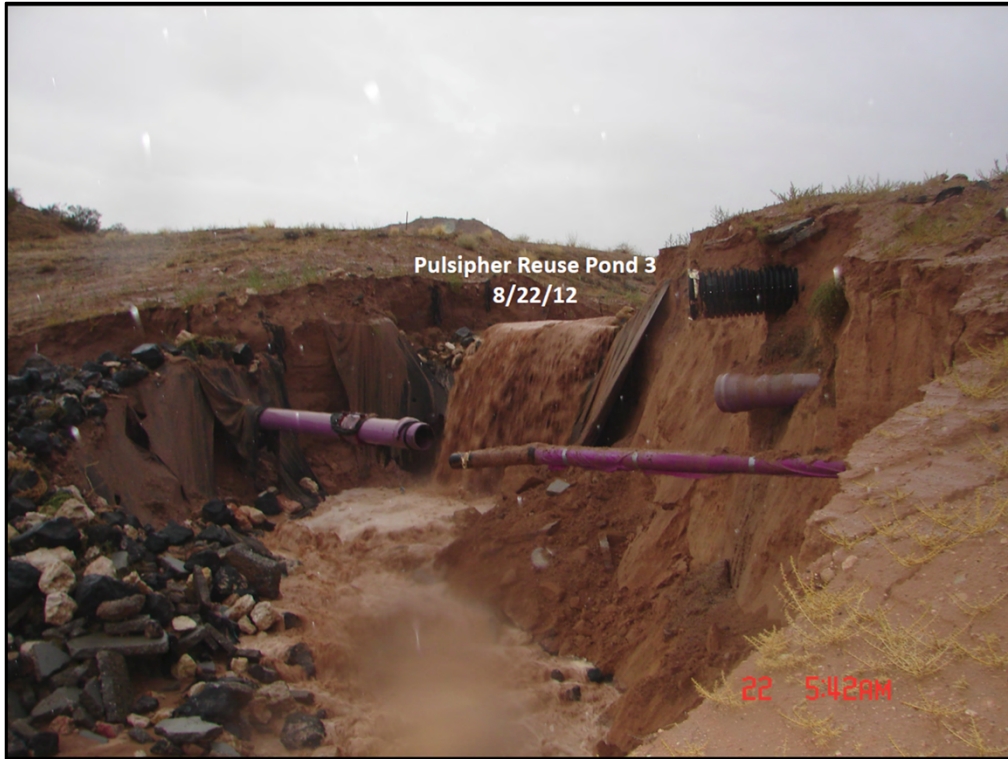
These reuse water lines were not in service at the time of the storm, but clearly they were damaged.
